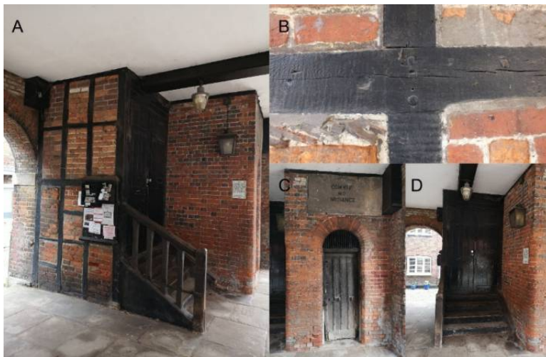
Figure 12 (A) Shows timber feature on interior of East elevation, showing staircase. (B) Shows detail of carpentry joint used to secure the beams with the pegs visible. (C) Shows the lock up next to the stairs still using Flemish bond with irregular burnt header bricks. (D) Image of original staircase.
