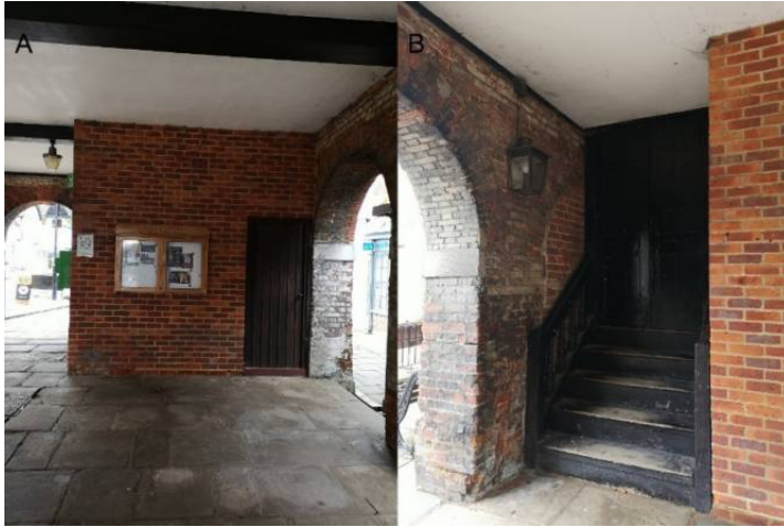
Figure 13 (A) Showing toilet block on West elevation (B) Showing new staircase added as part of 1911 renovations, you can see the scar of the arch just above the side of the staircase.
